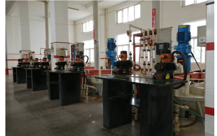
R&D Pilot Plant
